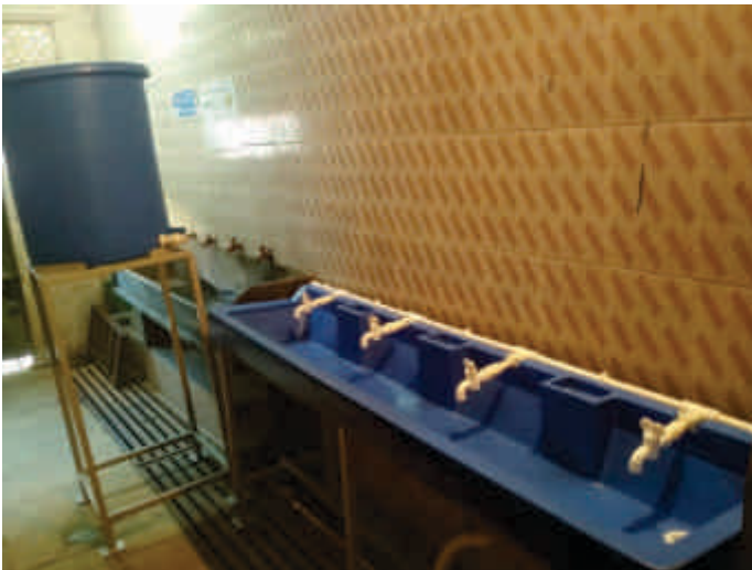
Hand Wash Station-Milind Vidyalaya-Powai
