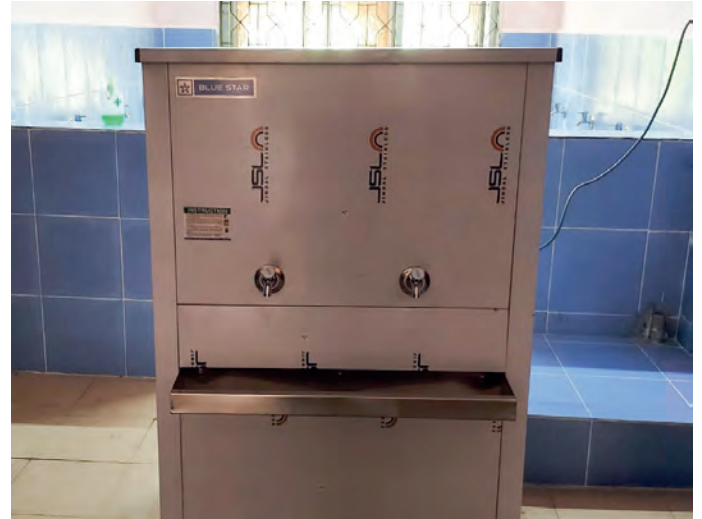
Water coolers (150 litres) setup in Motilal Nagar School, Goregaon West - Mumbai
